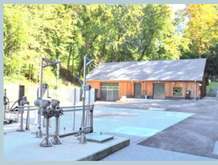
Station d'épuration Consdorf 4000 EH
