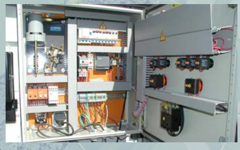
Station de pompage Dielchen
